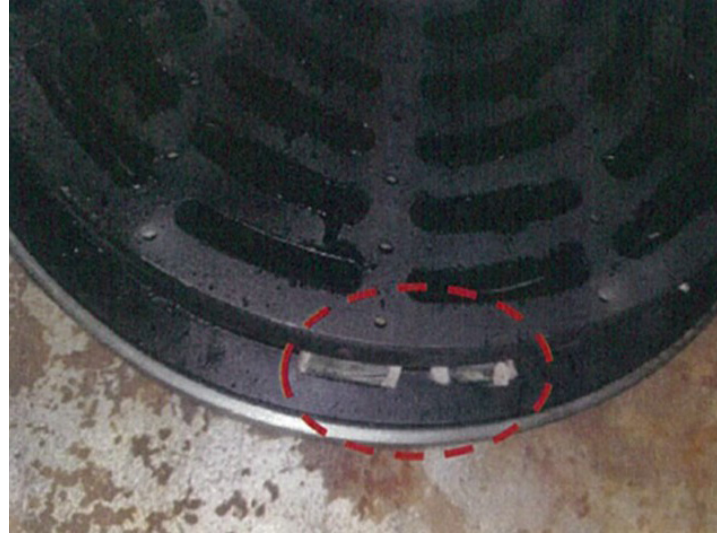
Figure 10. Damage on Ring Plate
