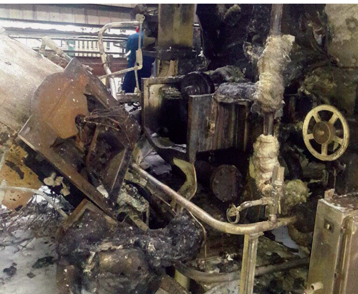
Figure 1 - Destroyed steam turbine due to overspeed
